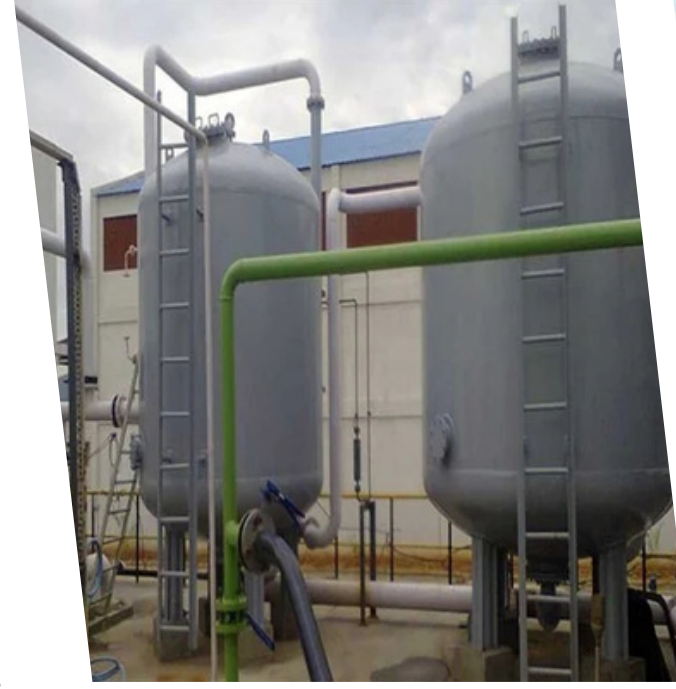
CONDENSATE POLISHING UNIT
