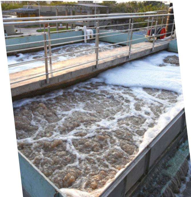
SEWAGE TREATMENT PLANT
