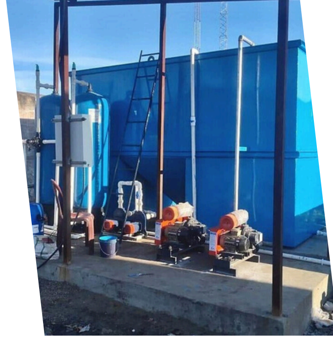
EFFLUENT TREATMENT PLANT
